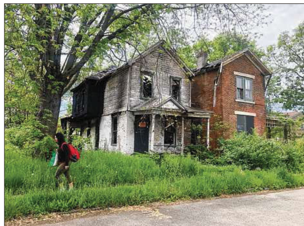
Fire-damaged homes at 2028 and 2030 East Fourth Street. The city is targeting the more severely damaged property for removal. CORNELIUS FROLIK / STAFF
